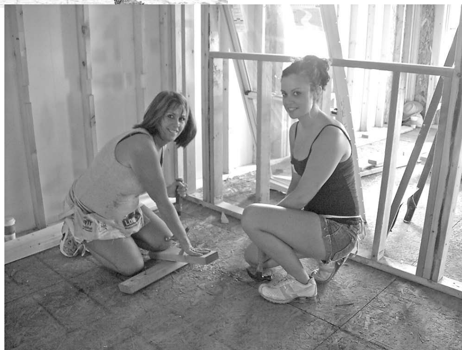
Photo by Habitat for Humanity of Monroe County. Habitat homeowner Paula Lawson and her daughter work on their home construction.
